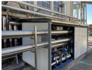
Indirect Steam Generator
