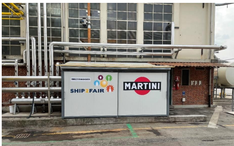
Image 2: Indirect steam generator
